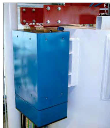
High current transformer, secondary connection
